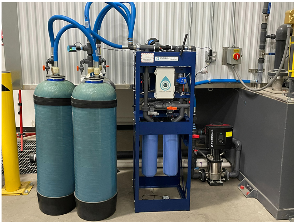
Figure 2. A Water One WX unit.
